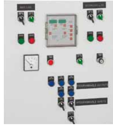
Control panel of a supply inverter with automation control unit Cat. N°. 0261 93
